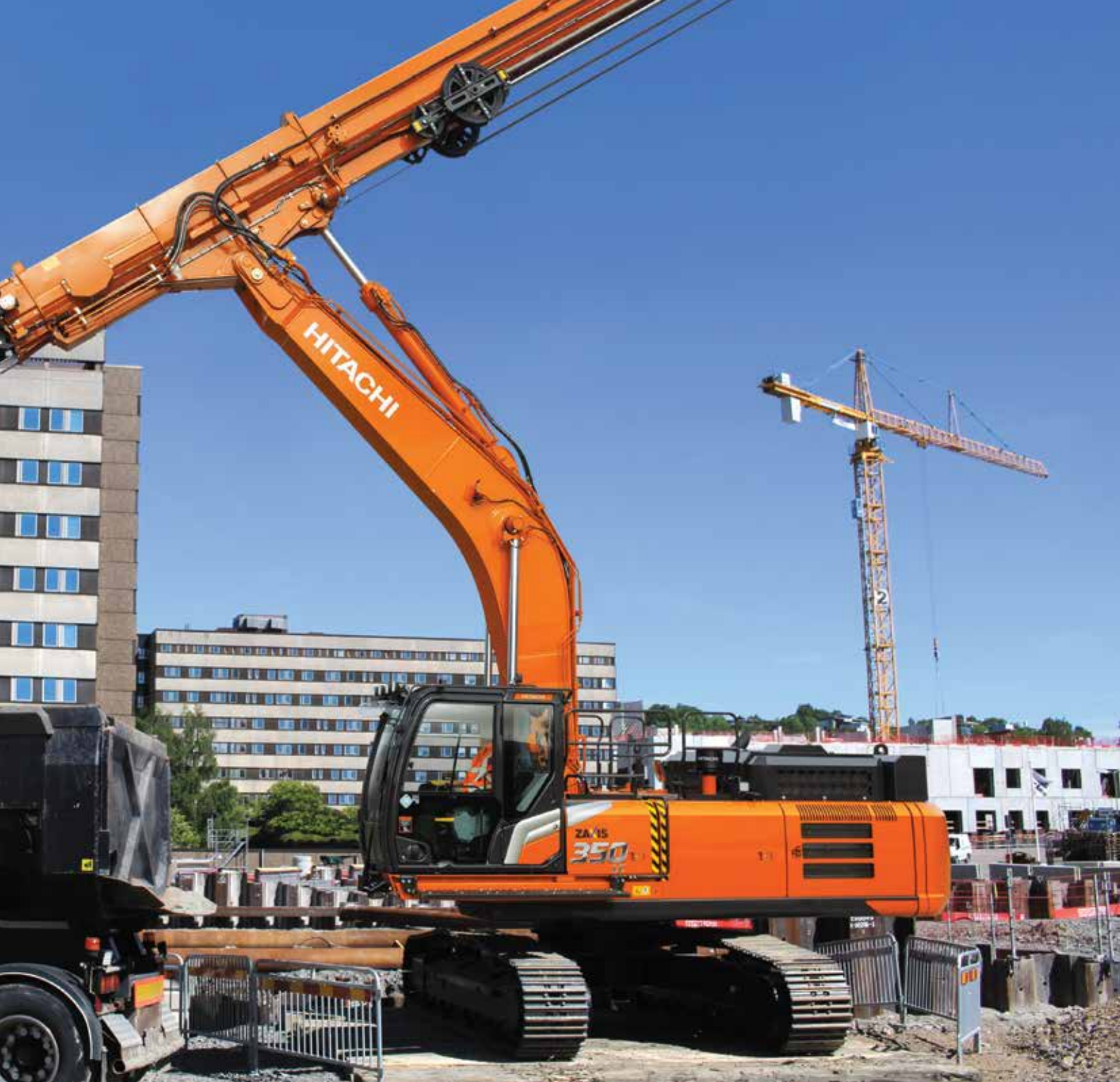
Removed soil can be loaded to trucks that transport materials swiftly off site.
